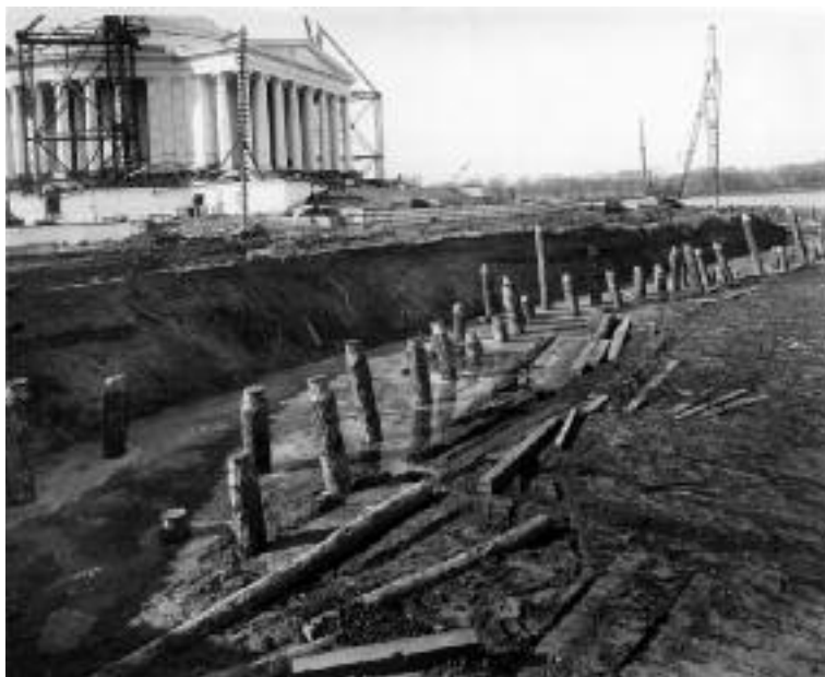
Timber Pile driving for original Seawall. What type and how long were the piles used for the Ashlar Seawall? Historic photo that answered this most important question. Notice start of pile driving in background.
