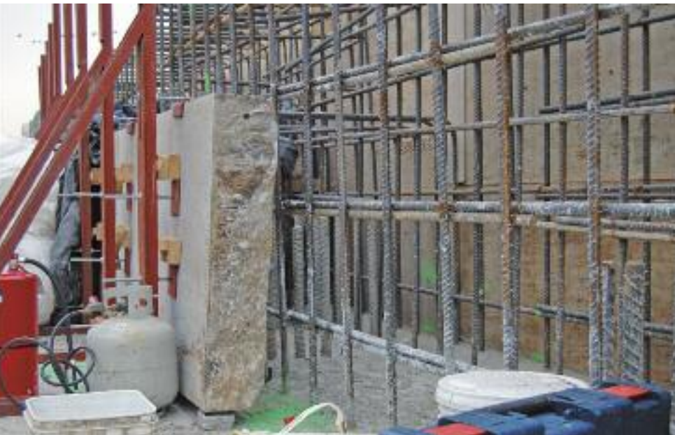
Original Ashlar facing stone re-positioned before pour of bottom section of the new wall stem.
