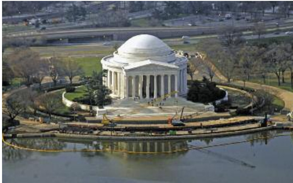
Construction activities on the North Plaza and Seawall at the Jefferson Memorial.
