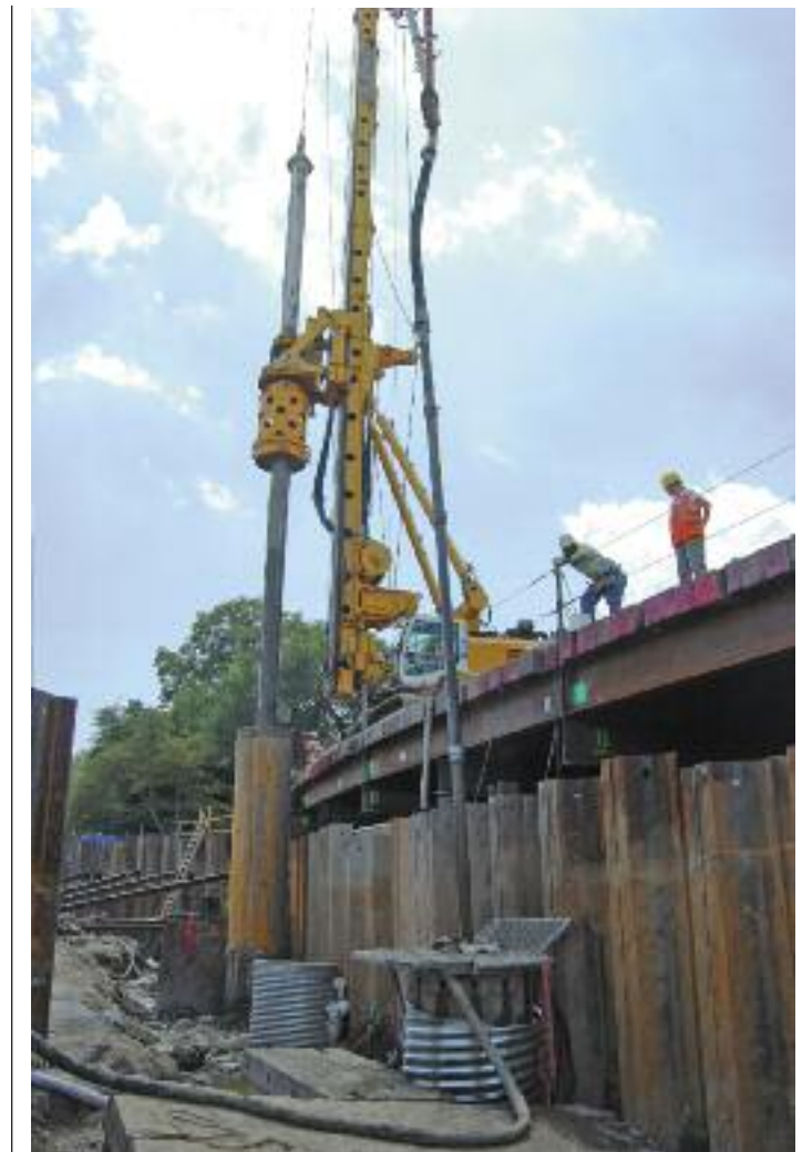
Caisson construction using the Bauer BG 40 (background) and caisson concrete tremie placement (foreground).
