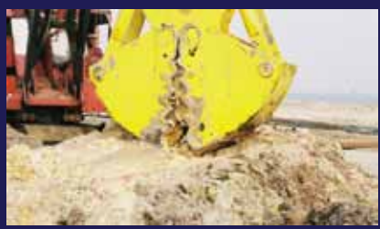
Excavating a Diaphragm Wall in Shore line Sands with Seawater Saturation and Tidal Influence
