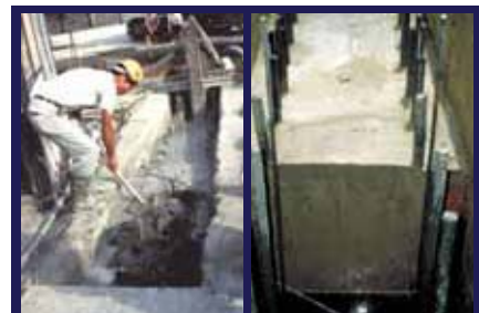
Concrete Rise Under Bentonite vs. KB Slurry on same project in Marine Clay
